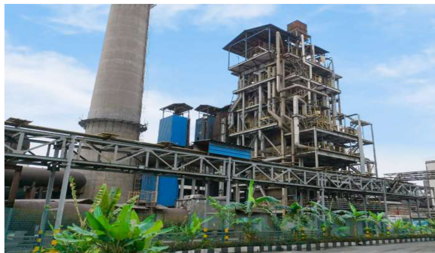
PT.IRNC 25MW 发电厂
